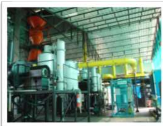
1.2MWe : Gujarat, India
