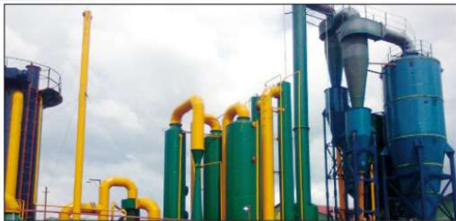
2MW CFBG POWER PLANT
