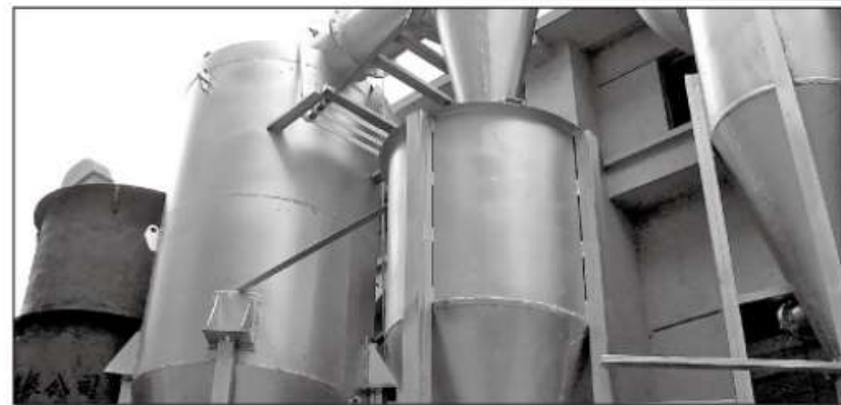
0.5MW CFBG POWER PLANT
