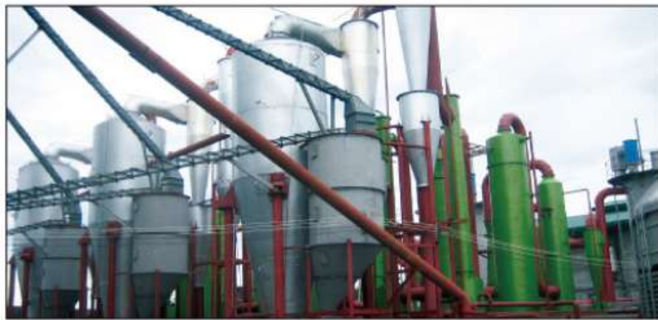
3MW CFBG POWER PLANT
