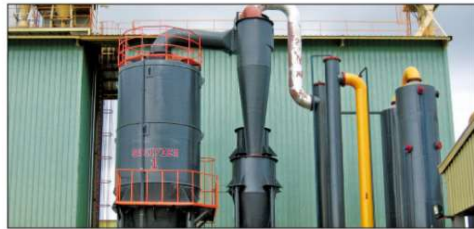
1.2MW CFBG POWER PLANT
